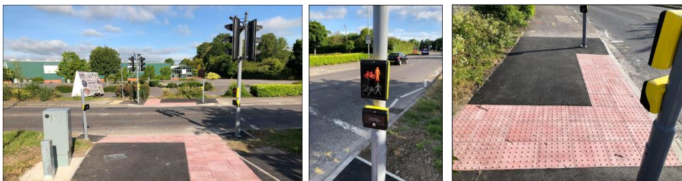
Aging traffic signals and pedestrian crossings are renewed as to keep them safe as here on the A350 at Melksham
