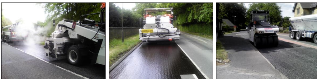
Surface Dressing programme start was delayed whilst safe Covid-19 compliant working processes were put in place, but continued as planned during the summer
