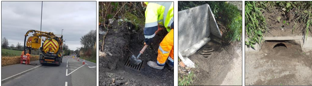
Keeping drainage systems clear and in working order is important all year round
